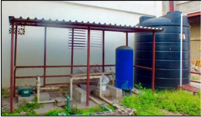
Water tank & Pump
