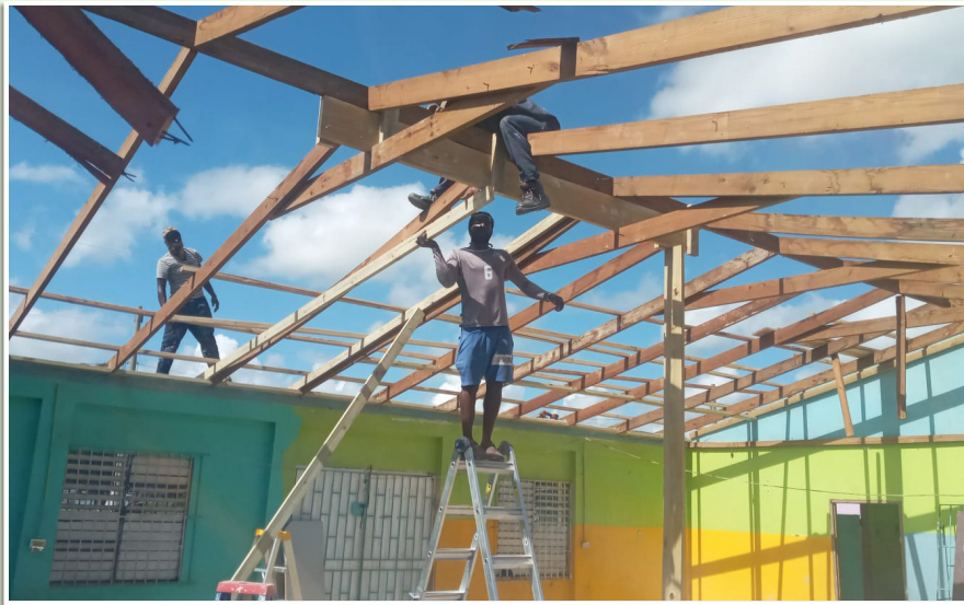
1. Contractors are hard at work to repair the roof of the Irish Pen Basic School as part of Sagicor Foundation's Adopt-A-School Programme.
