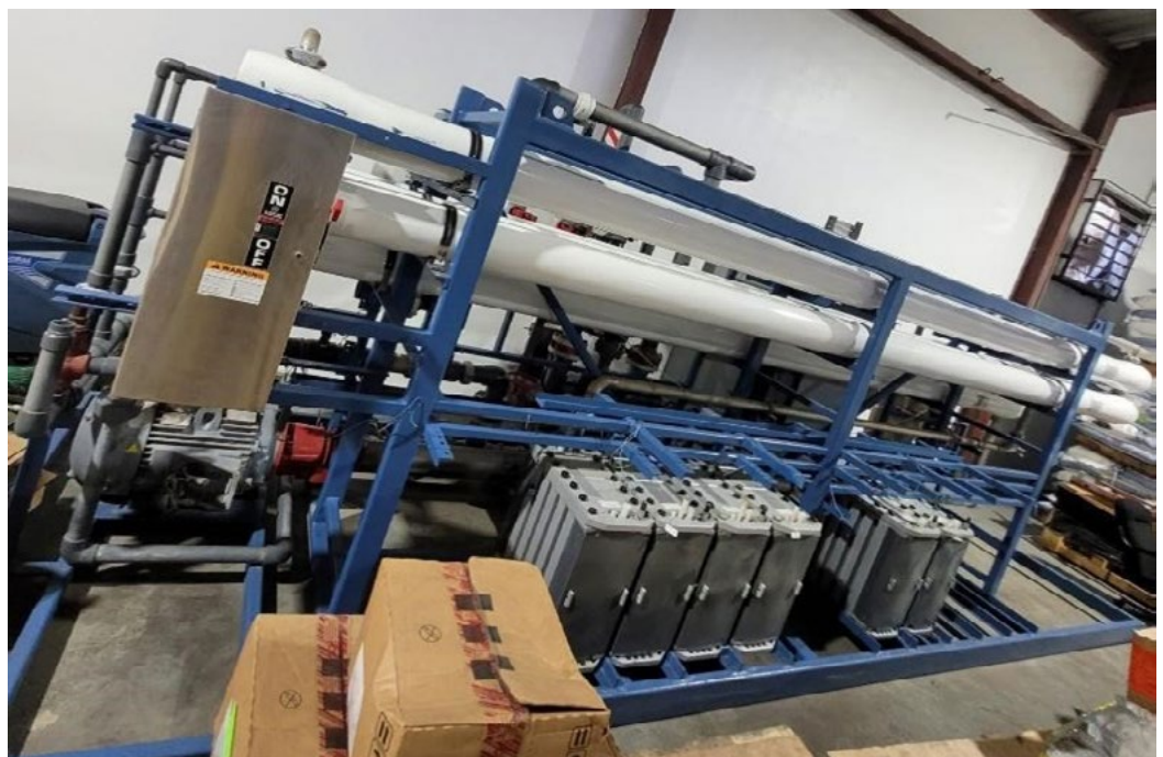
Reverse Osmosis Plant
