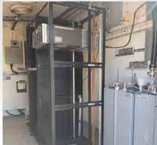
Figure 4 – New 94.1 transmitter at the Kensington Transmitter site, Portland.
