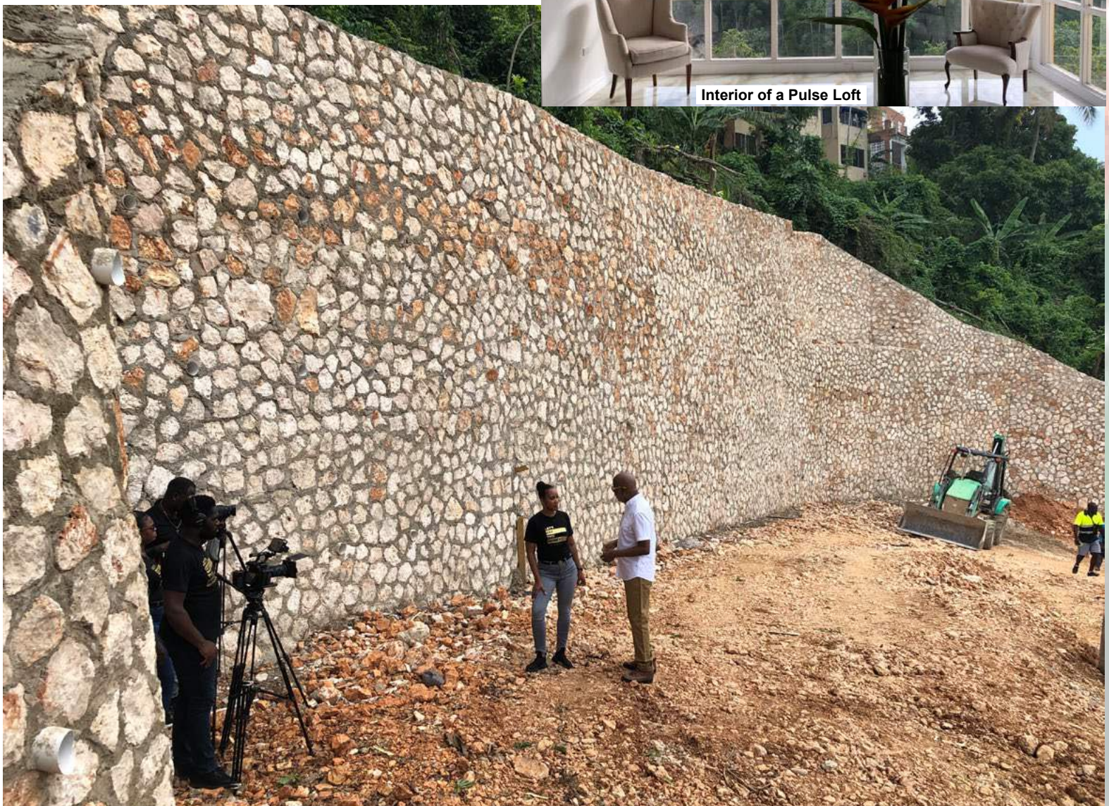
Kingsley Cooper and Kailah Reynolds of KR Media in discussion at Pulse Lofts as he outlines plans for the completion of the roadway and parking lot.
