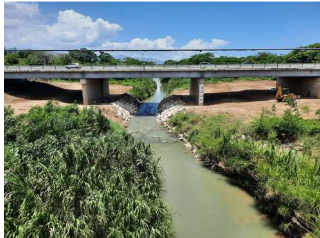
Rio Cobre – cleaning of channel as well as replacement of missing riprap
