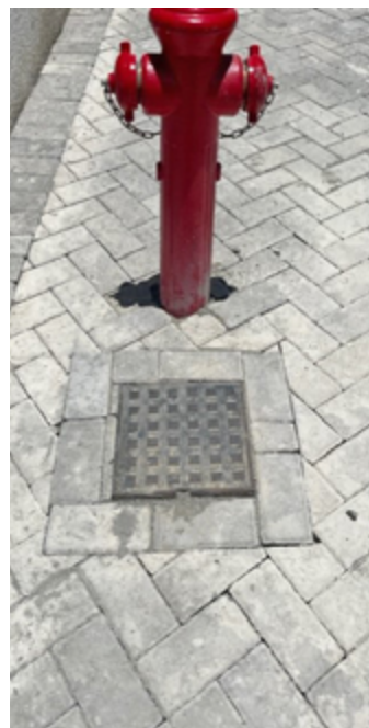
Figure 5b: Fully commissioned fire hydrant.
