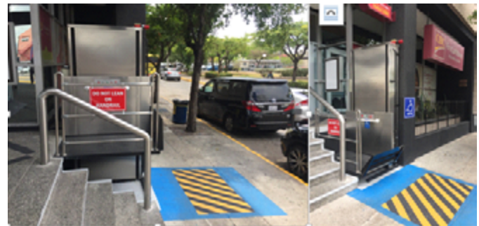
Figure 6: Wheelchair Lift intalled at FCIB building in New Kingston by Comfortair Engineering Ltd.
