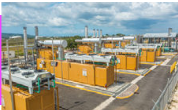
A view of the JPS 10MW Combined Heat & Power (CHP) Plant providing electricity and steam to the CB Group's processing plant.
