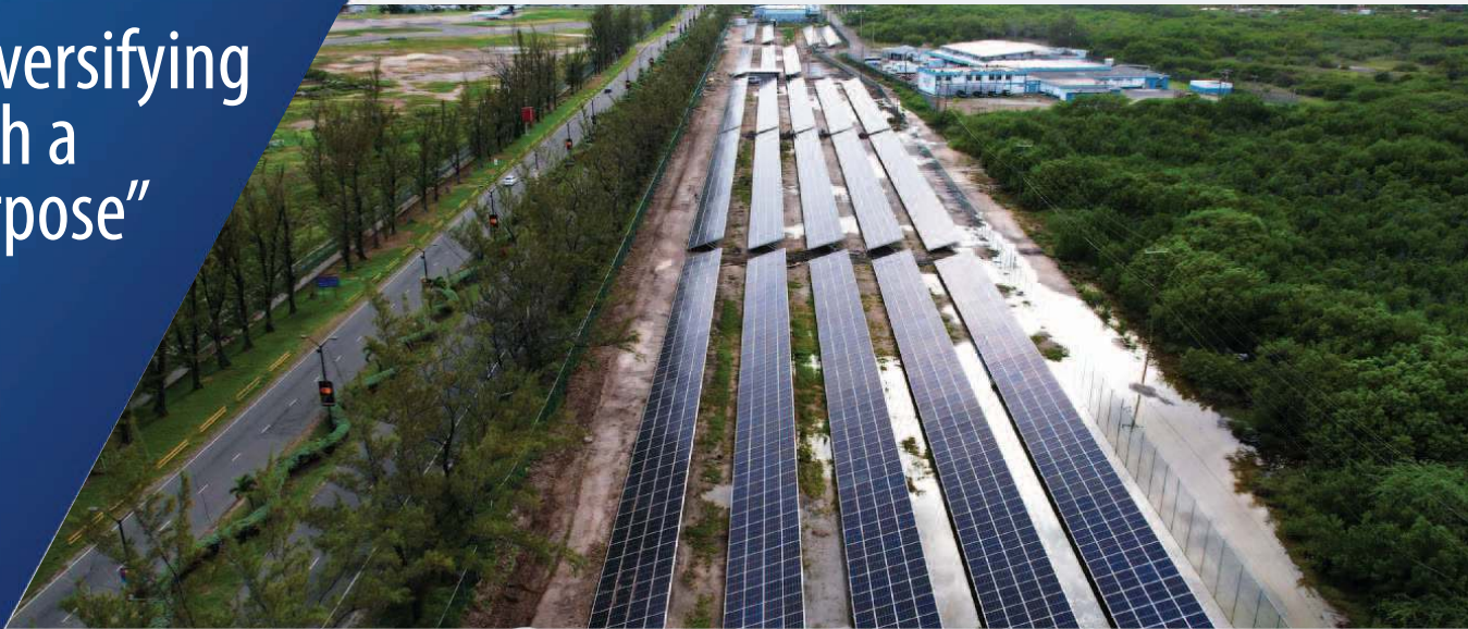
The Norman Manley International Airport, Jamaica goes solar through this 2MW solar photovoltaic installation that was completed by IEC SPEI Limited and Wigton.
