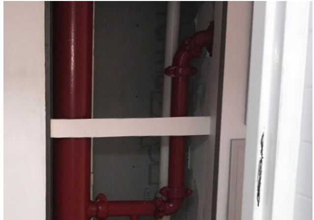
Wet Riser supply system for the distribution of water to the respective floors of the Scotia Centre building, a key component of the firefighting systems
