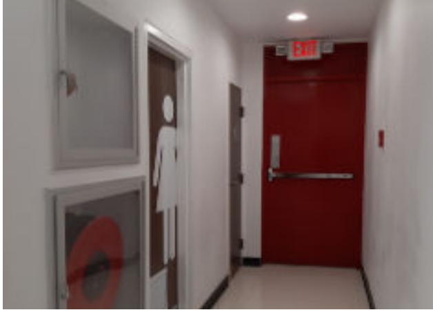
2-hour Fire Resistant Emergency Exit Door with updated exit signage; updated fire cabinet with new fire hoses and new extinguishers
