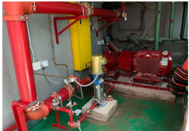
Newly installed fire pump - an essential component of the building's fire protection system, especially in high-rise structure
