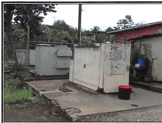
View of telecommunication equipment
