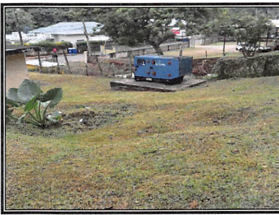
Generator on subject site
