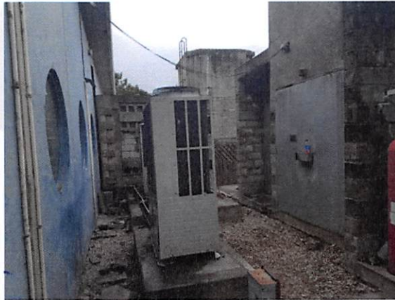
Gen & switch room
