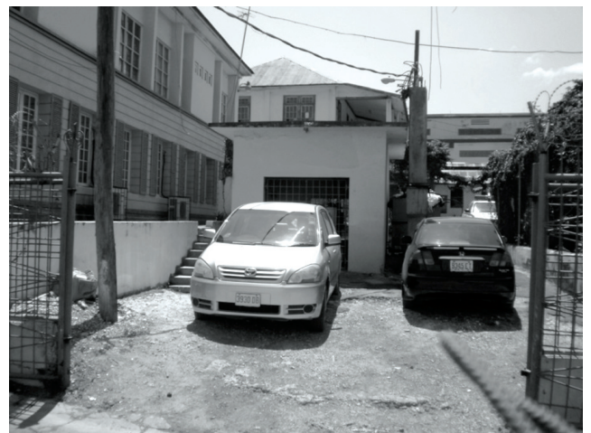
Generator & Parking Lot
