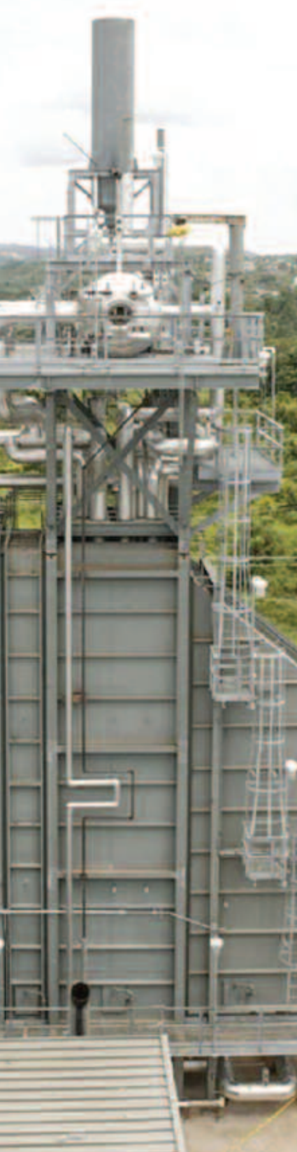
Bogue Power Station
