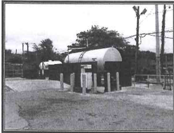
Diesel petrol pump
